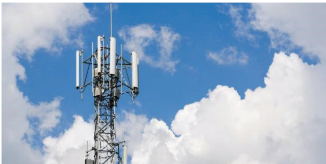
Antenna Tower (Source: NYU)
